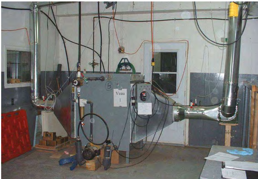
Figure 3. A picture of the air cleaning system.
